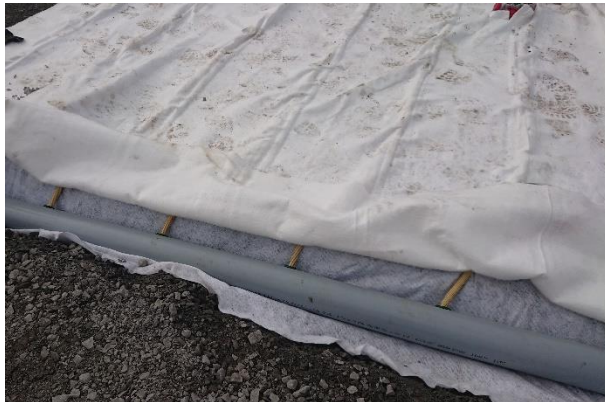
Figure 9. Single connection to the header pipe
