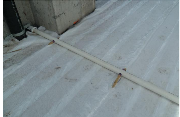
Figure 10. Double connection to the header pipe
