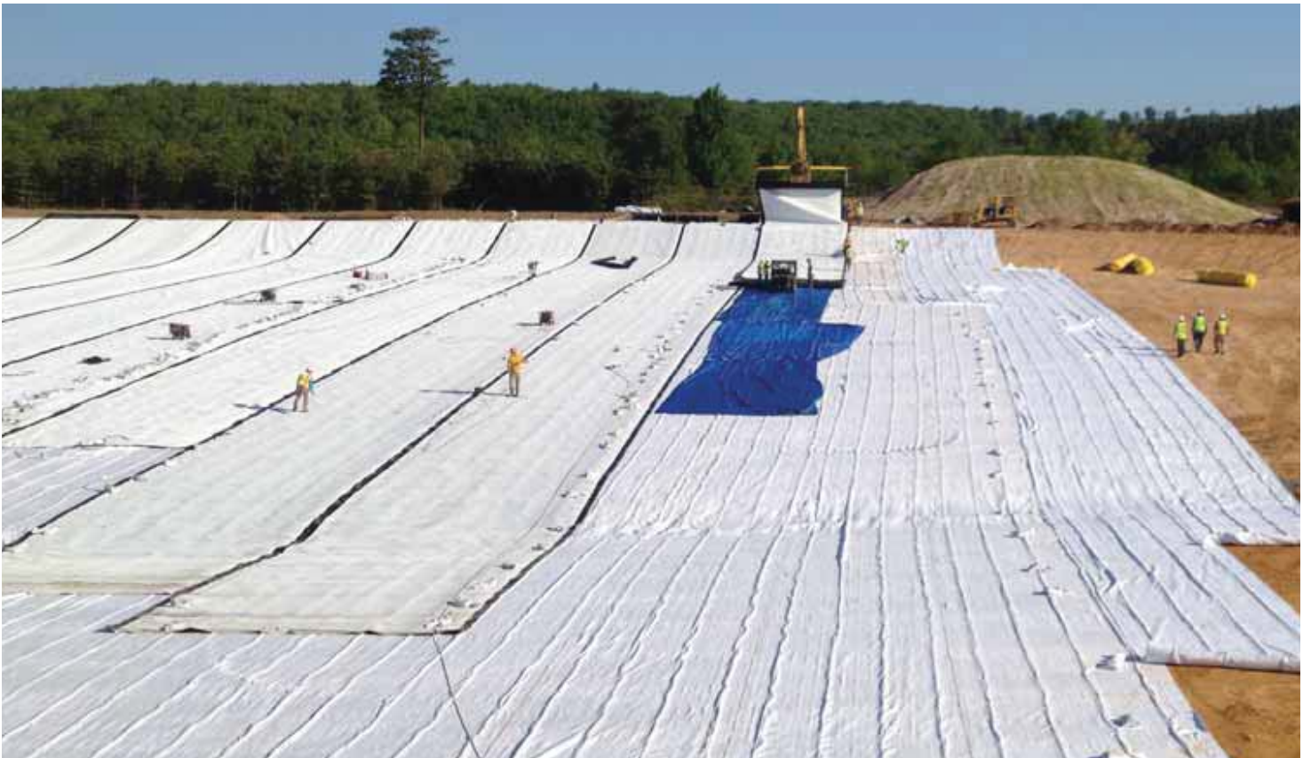
FIGURE 3 Installation of an exposed, 1.5 mm (60 mil) HDPE liner underlain by a draitube geocomposite.
