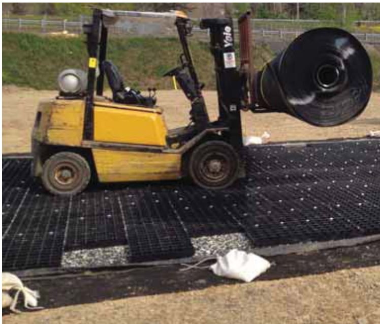
FIGURE 5 A well pad system that consists of, from the bottom up: a 1.5mm (60mil) HDPE textured geomembrane, a 340 g/m 2 (10 oz./yd 2 ) cushion geotextile, a 50mm (2in.) recycled foam product, and a durable, reusable specialty mat product.
