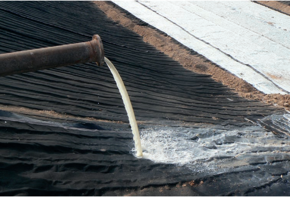
FIGURE 2 Multilinear drainage geocomposite used in a slurry dewatering facility. Photograph courtesy Afitec-Textel
