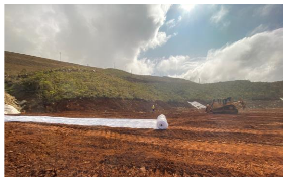
Installation of DRAINTUBE 300P FT4 D25 in strips on the surface of the platform.
