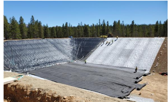
Installation of DRAINTUBE 606 ST1 D25 as leak detection layer between the primary reinforced polyethylene geomembrane and the geosynthetic clay liner.
