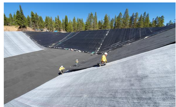
Tacking of the DRAINTUBE® on the GCL. The multi-linear geocomposite provides an additional cushion for the overlying geomembrane.
