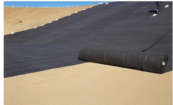
DRAINTUBE 606 ST1 D20 installation for gas collection under the secondary geomembrane. DRAINTUBE® is connected to the main header pipe using the Quick Connect System.
